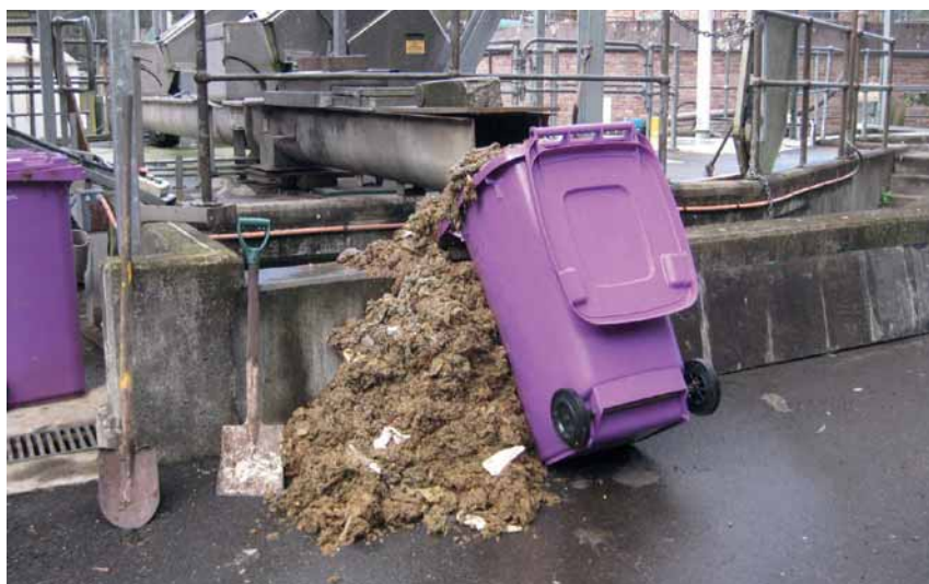
The impact on the environment can be dramatic, with overflows caused by sewer blockages contaminating local creeks, rivers and even beaches.
