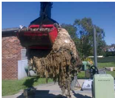
An example of the destructive nature of wipes in our pipes.
