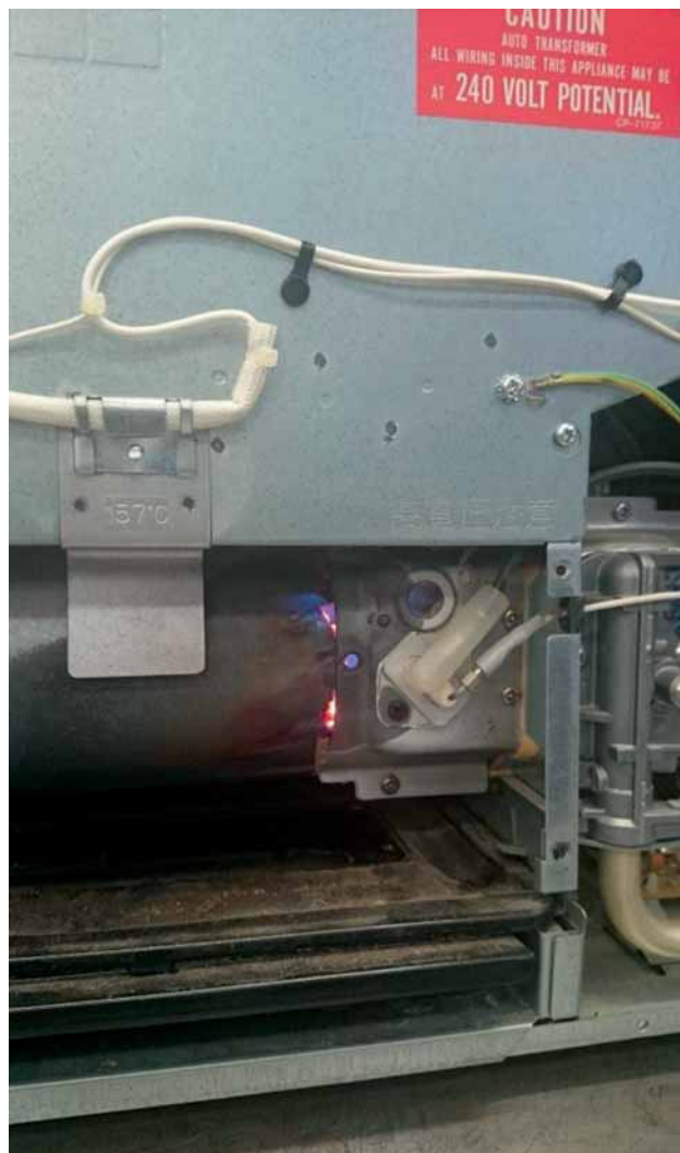
This heat exchanger is still in operation, despite two obvious holes appearing.
