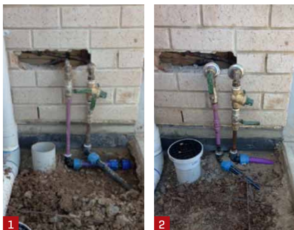
IMAGE 1: Before: cross connection. IMAGE 2: After: no cross-connection.
