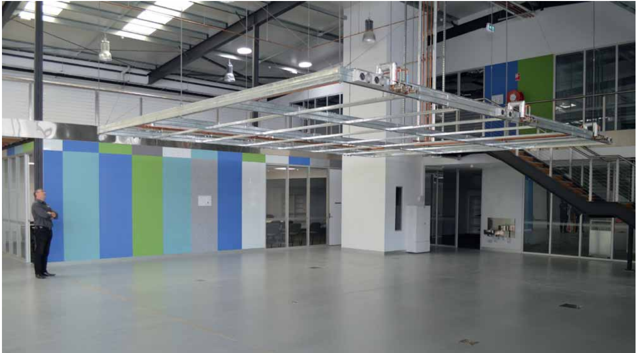
The construction itself is completed in Geelong and is now at the fit out phase. PICAC estimate that it will be delivering training in the coastal city by mid to late this year.
