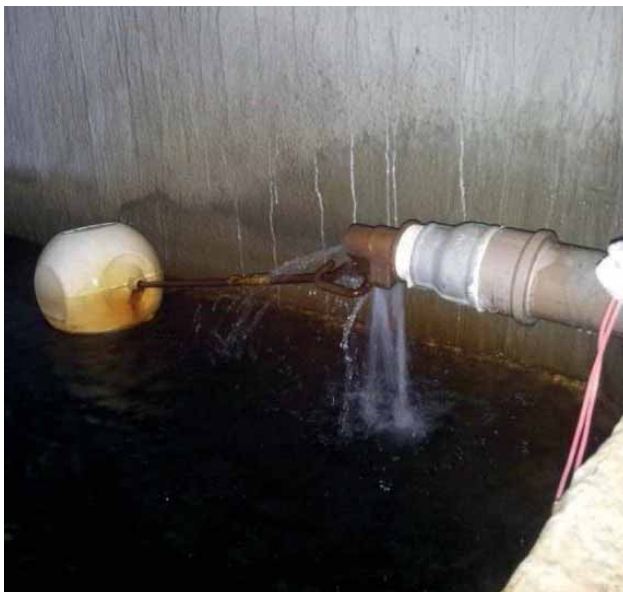
The above is a typical installation of mechanical float valves.
