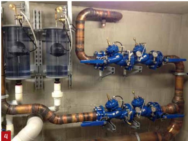
IMAGE 3: Level control of emergency fire protection reservoirs in buildings. IMAGE 4: Be sure to always install WaterMarked and/or Australian certified products.
