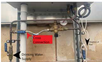
Image 1: The flexible connection is the 'quick-fill' that should be disconnected and capped once the system is full.
