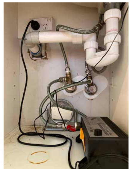
Non-compliant Flexi Hoses cause millions of dollars' worth of damage to Australian homes every year.
